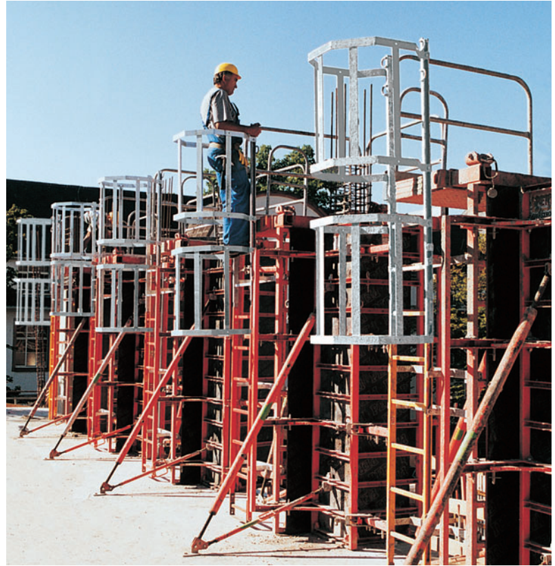
Ladders for safe access of the platforms.
